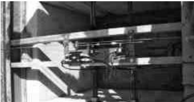
Electrical monitoring device
